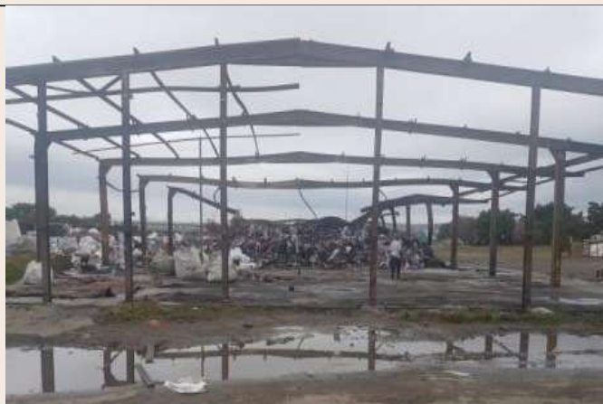
A: Burnt overhead structure
